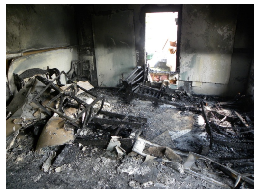
The aftermath of one of the apartment units burned for research. ATF installed cameras inside to each unit to monitor fire progression as it relates to ventilation. Afterwards, arson investigators used the scene for training purposes.
