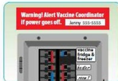
Label fuses and circuit breakers. Post a sign to alert the Vaccine Coordinator any time the power goes out.
