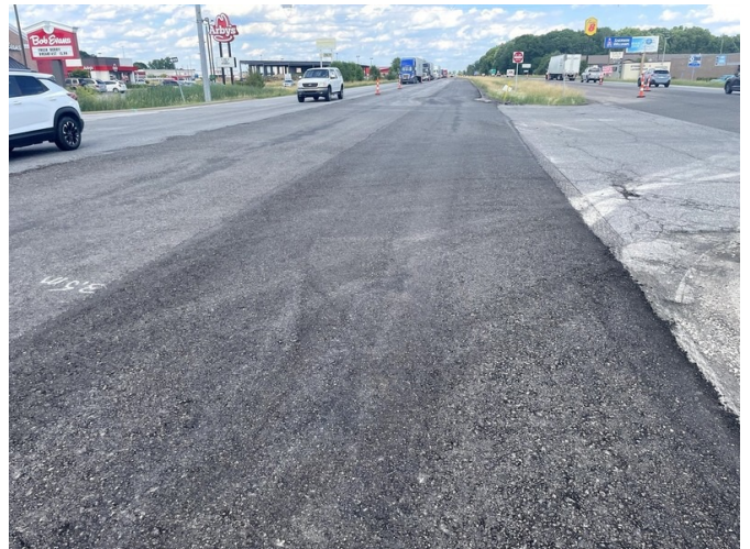
Due to heavy traffic volumes, the CIR mat was opened to intersection traffic directly after compaction with little to no raveling observed
