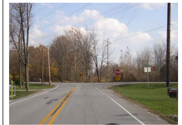
Passing restrictions and minimal access control are the primary limitations to capacity on SR 32.
